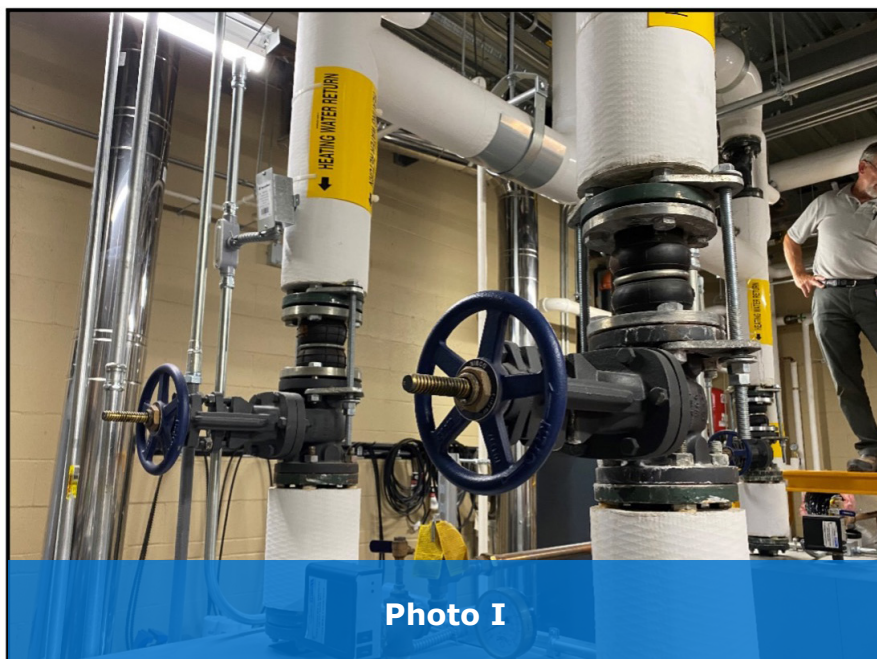
Photo I. Example of Insulated Pipes in Existing Greenhouse
